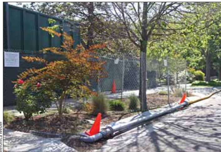
Groundwater is pumped from a construction site on Webster Street down to the block's storm drain in April.
