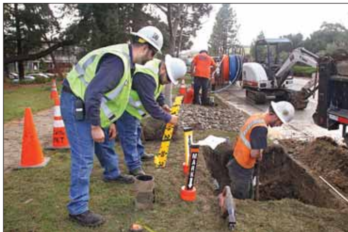
Kenny Zertuche, far left, and Manny Martinez, left, field service representatives with the City of Palo Alto Utilities Department, survey a broken gas line on Page Mill Road on Feb. 9.
